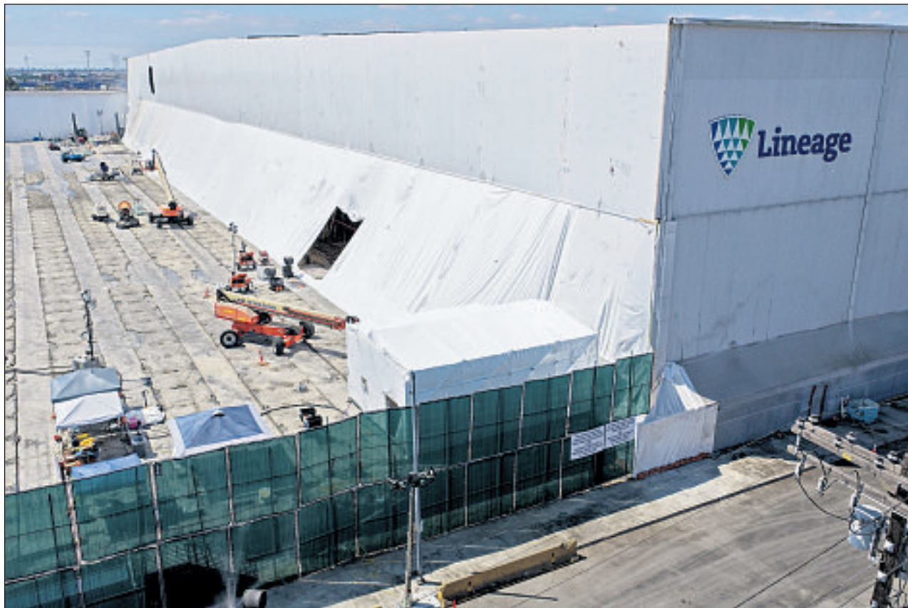
IN BOYLE HEIGHTS, crews continue cleanup efforts after a June blaze engulfed a cold storage warehouse. ALLEN J. SCHABEN Los Angeles Times
