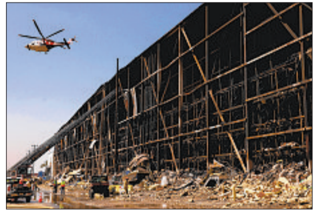
A HELICOPTER finishes a water drop at a cold storage facility that has burned for more than a week. GENARO MOLINA Los Angeles Times
