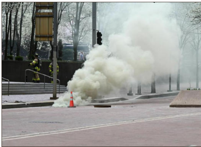
Smoke pours out of a manhole on Grant Street on Tuesday after high voltage wires caught fire, causing a pressure buildup that led to explosions in Downtown Pittsburgh.
