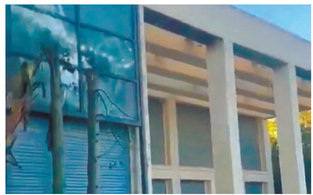
Damage to Netanyahu's Caesarea home from the drone. Used in accordance with Clause 27a of the Copyright Law
